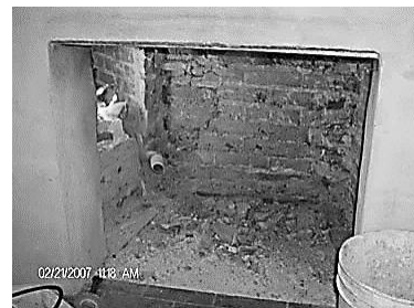
Badly Deteriorated Firebox
