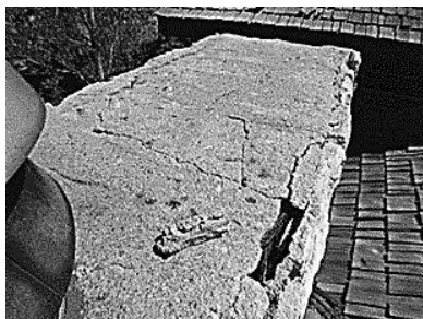
Damaged Chimney Cap
